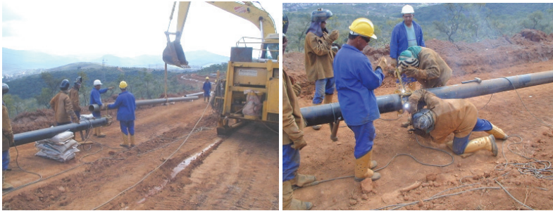
Fig. 29. Preparation of a pipeline assembly. (a) pipes positioning and (b) root pass.
